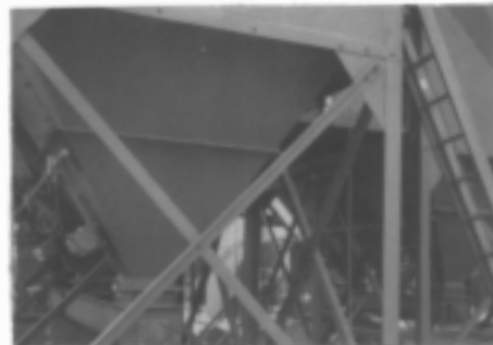
2P-200 on Dust Collector Hoppers
