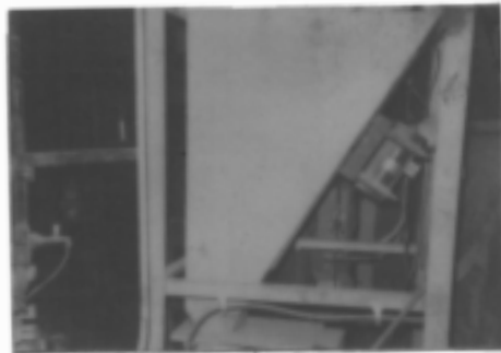
Vertically mounted 2P-450 on Crushed Cullet Hopper.
